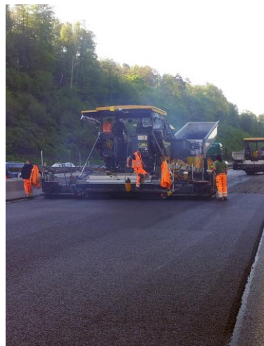
process optimisation, temperature data and documation are getting more and more important in road construction
